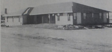
NOW UNDER CONSTRUCTION located on the far western edge of Clarendon is this beautiful new home of Dr. and Mrs. Chas. E. Deyhle.
