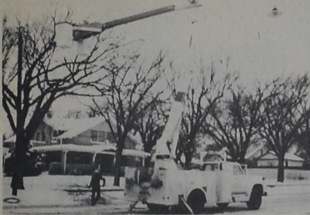
WEST TEXAS UTILITIES service men repair broken power line leading to James F. Hayes' home.
