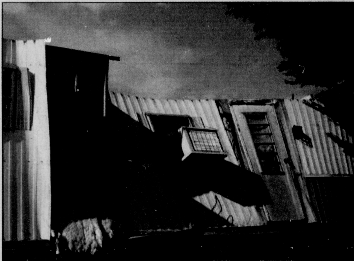
D.W. Rankins trailer house on Swanson Street was heavily damaged by high winds that struck the City of Howardwick Monday night. Damage across the city varied from moderate to severe, but residents are thankful no one was hurt during the storm.
