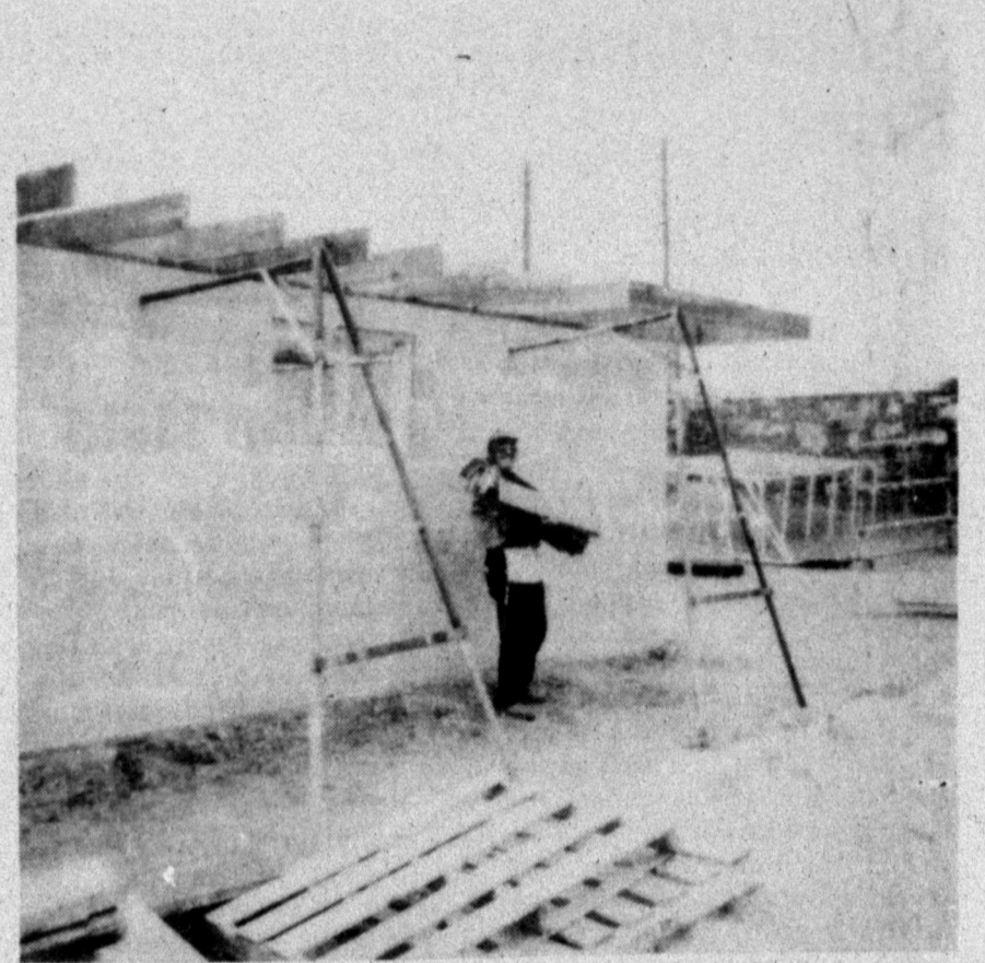
TEDDY ASHCRAFT busy at work on the new Weight Lifting Room at Bronco Stadium.
