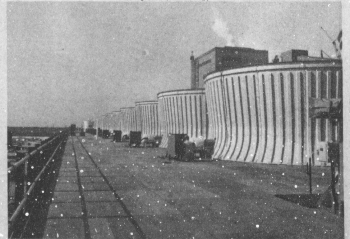
COOLING TOWERS-- A dozen giant fans pull air up through one of the two "cooling towers" at Southwestern Public Service Company's Tolk Station Unit No. 1. Each cooling tower works just as an evaporative cooler at a home does. The towers lower the temperature of water, which is used--and reused as many as five times--in the electricity generating process at the coal-fired plant. (SPS PHOTO)
