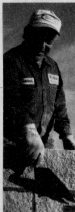
Clarendon Junior High Principal Marvin Elam and contractor Roy Williams (center) position reinforcement bar for the foundations of a dugout at McClelland Field assisted by sophomore Steven Ballard. Left: Gabriel Camacho lays cinderblock for the west dugout at the new softball field. Enterprise Digital Photos
