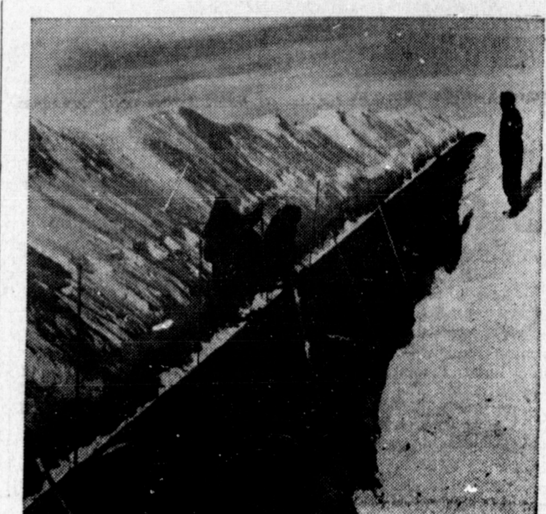
MODERN U.S. ARMY ingenuity fashions an entire camp under Arctic ice and snow. Here, members of the U.S. Army Polar Research and Development Center work on a permanent camp in the Far North. Men are placing pipes through the corrugated steel arches at regular intervals to leave holes for wiring and plumbing. Snow will be blown over the arches and arches will later be removed, forming a roof of ice.
