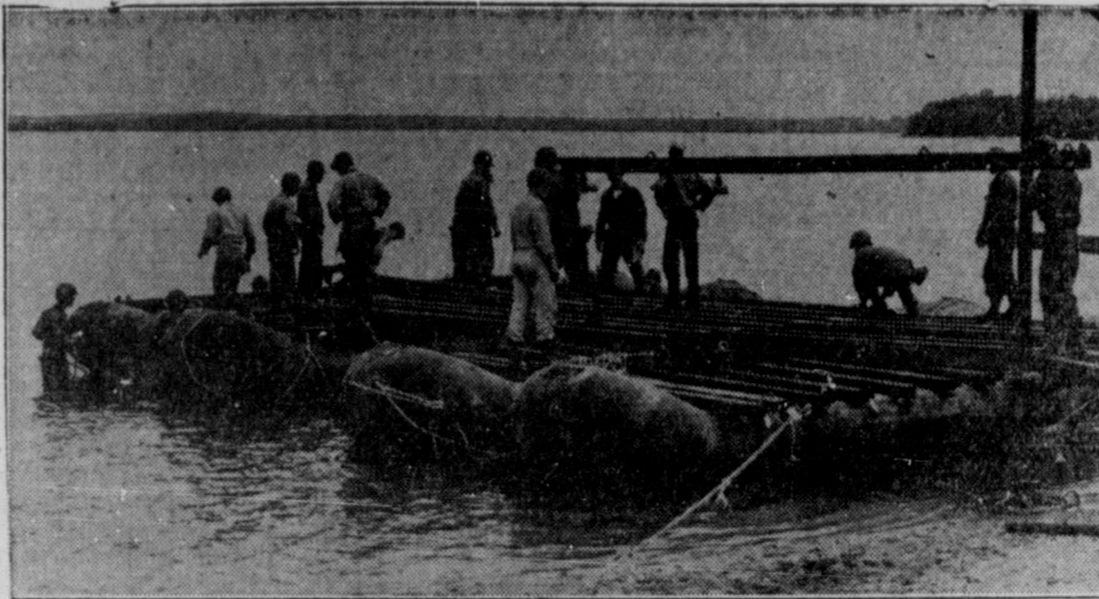
FAST WORK BY NATIONAL GUARD BRIDGE BUILDERS—Members of the 1806th Engineer Aviation Company, Dearborn, Michigan, and the 1427th Treadway Bridge Company, Sault St. Marie, Michigan, combine their equipment and talents in the erection of a pontoon bridge during summer field training of the 46th Infantry Division of Michigan at Camp Grayling.
