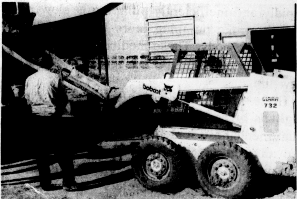
RONNIE BAKER was the contractor for pouring the cement floor in the new community center.
