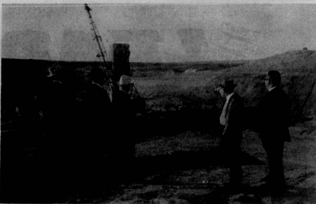
WORK ON THE LAKE GREENBELT reservoir is being inspected here during the stages of construction by directors of the greenbelt Municipal and Industrial Authority. Left to right are Merl Kincaid of Crowell, Wendall Harrison of Memphis, Bill Lowe of Clarendon, the job engineer, Mr. Alexander, and Carroll Knorpp of Clarendon.
