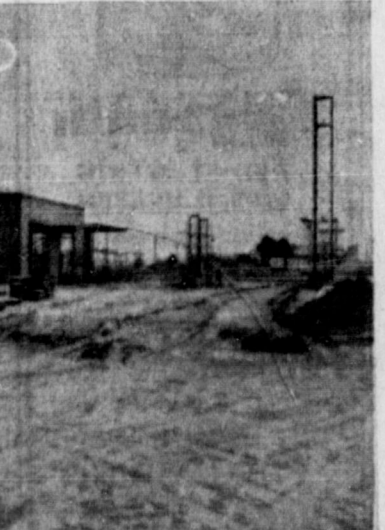
Construction In Progress—Photo at left shows the new T & M Oil Company station and warehouse as construction progresses. The tower in front will hold the big Phillips 66 sign in the crate at left. John H. Jones is the contractor. Photo at right shows bulldozer digging hole for big storage tanks for the new Airspeed Oil Co. station which will be constructed across the street east of Landers and Ray Super Save. It will be a Kerr-McGee station with the trade brand of Deep Rock. The building lot was leased to Airspeed by Lloyd Risley, who recently purchased the property from the Geo. B. Bagby Estate.
