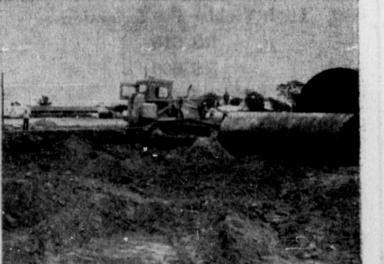
Photo at right shows bulldozer digging hole for big storage tanks for the new Airspeed Oil Co. station which will be constructed across the street east of Landers and Ray Super Save. It will be a Kerr-McGee station with the trade brand of Deep Rock. The building lot was leased to Airspeed by Lloyd Risley, who recently purchased the property from the Geo. B. Bagby Estate.
