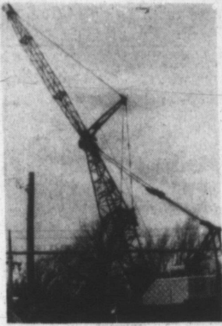
Construction has begun for a new water tower for the city of Hedley.
