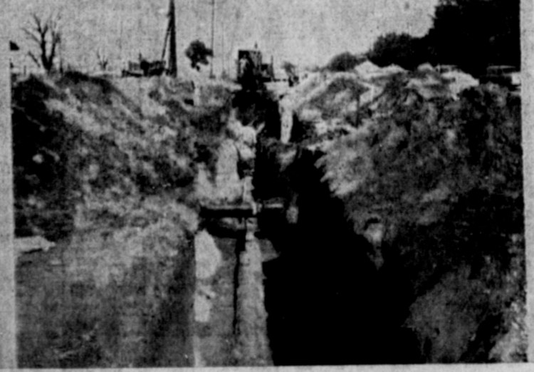
right shows the big pipe coming of Foxworth-Galbraith Lumber Co. The 14 inch pipe hit its biggest problem here, that of going
