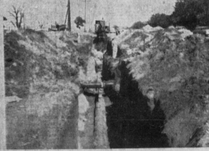
of Foxworth-Galbraith Lumber Co. The 14 inch pipe hit its biggest problem here, that of going underneath the tracks and crossing the city ditch, but it only had to travel around 1500 feet to completion.
