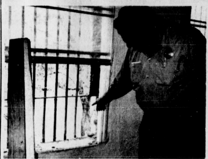
Police Chief Gary Gerdes points to where jailbreaker removed iron mesh, kicked out brick within an hours time to escape our county jail Wednesday afternoon. If we are to hold prisoners after taken into custody, we need a more modern facility than we have now was the comment of Gerdes and Sheriff Frank Lindsey. Staff Photo
