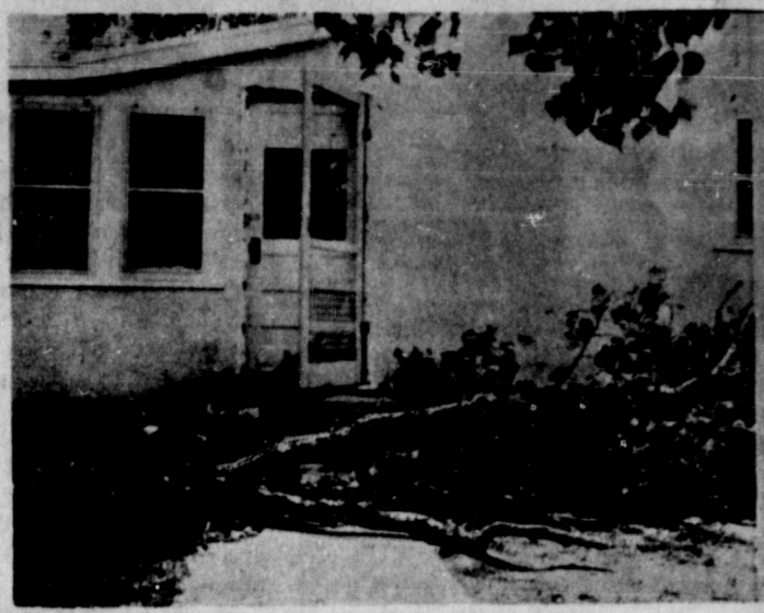
This big Cottonwood limb disrupted the peace and quiet at the home of Mrs. Edna Osburn Saturday night. The storm which blew thru broke the limb and drove it through the back door. Water damage to the home was high... and Edna, after going thru the tornado a few years ago at Martin, was quite shook up. Staff Photo
