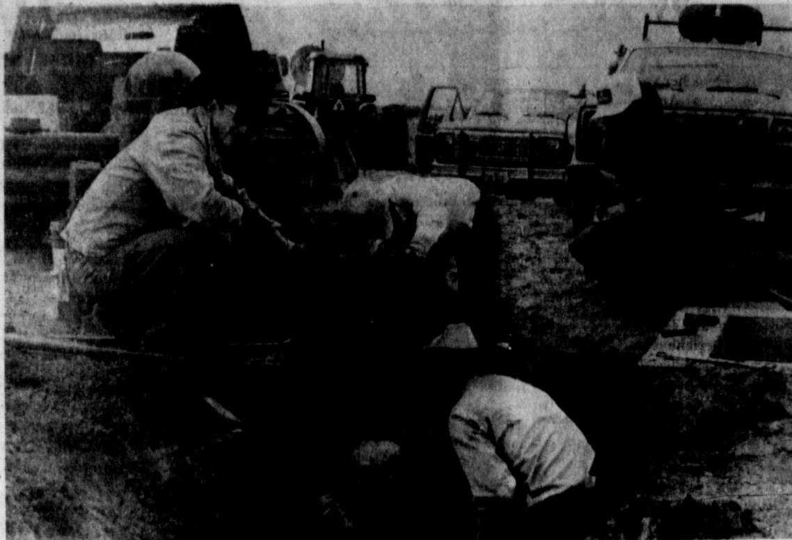
DANNY ASKEW watches as City of Paducah installs a Care-Free water conditioner.
