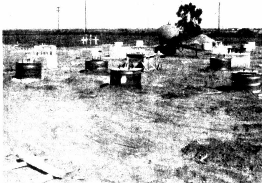
WORK PROGRESSES on the Thunder Junction site north of Clarendon. Shown here are the concrete foundations for the waterslides.
