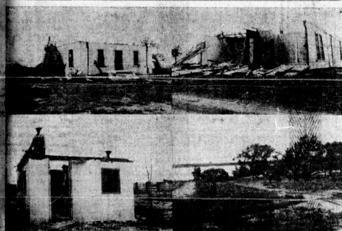
Pictured top left is Raymond Farr place near highway 70; right—M. G. Helton place west of the J. D. Jones home. It was being remodeled so they could move back from Pampa. Bottom left, Slaton, Frank and Ed Mahaffey doing a repair job on outbuilding at Ed Mahaffey place. Ed said he saw 20 or more funnels drop down out of the cloud. Right is Jack Breswell home on Forrest Sawyer farm just north of town, showing the growth of what was once a small pond. Only a few hundred yards separate this lake from the Bugbee lake to the west which now covers many acres of good farm land.
