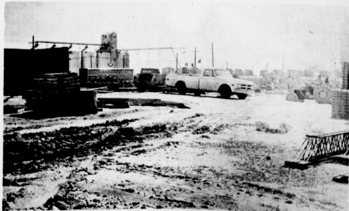
CONSTRUCTION PROGRESSING ON BANK. . . Construction on the new bank building for the Muleshoe State bank, located at the crossroads in Muleshoe is progressing on schedule and maybe a little ahead of schedule, according to bank president Bill Loyd. Completion is scheduled for early November on the new, larger bank building. Walls are now going up with the completion of the foundation.
