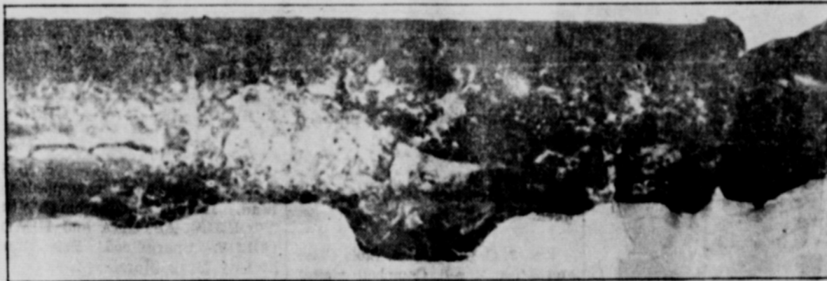
Above: Wire with insulation blistered. Such heating causes energy losses of as much as 25 per cent of light bulb or electric appliance efficiency.
