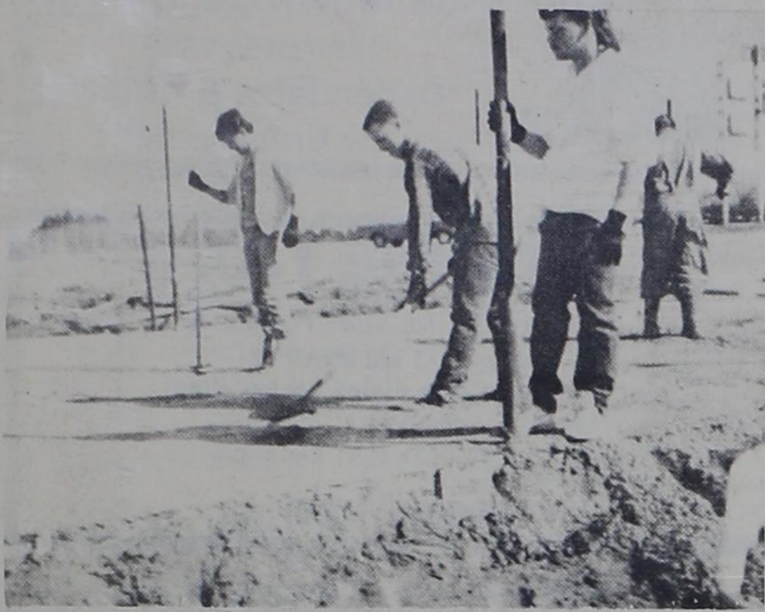
PITCH IN — Four of Cross Plains' Ag students are working on the freshly poured cement for the new concession stand. (From left) Darin Apple, Ken Masters, Dave Wilson, and Billy Bell.
