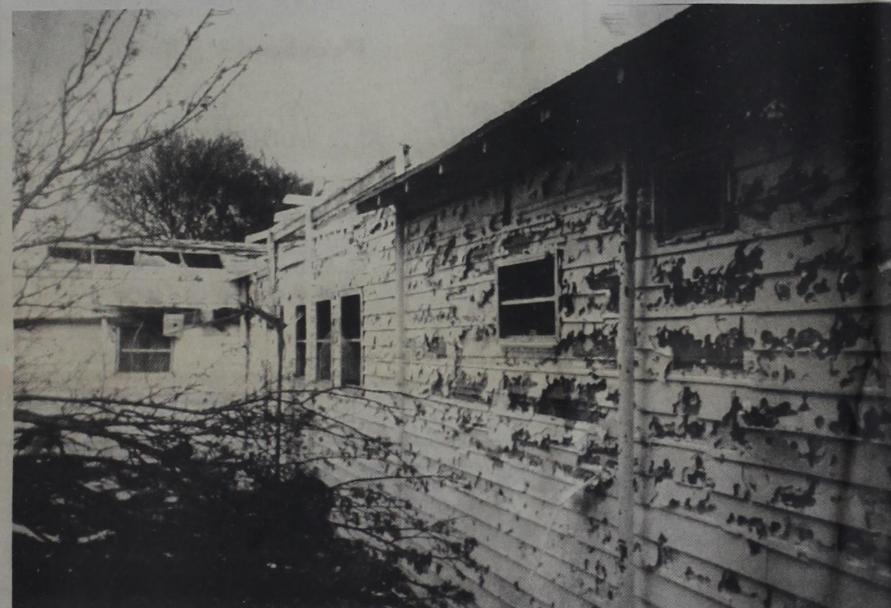
HAIL PEELED THE PAINT FROM THE DRAPER HOUSE
