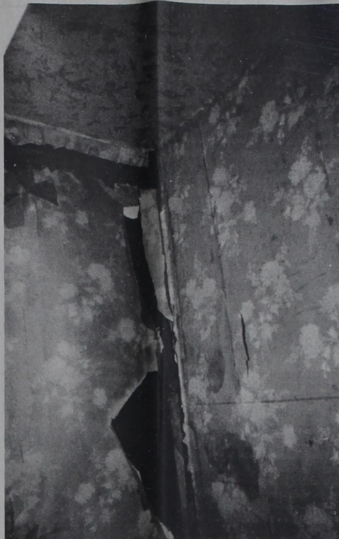
WALLS CRACKED INSIDE THE GLENN CHAMPION HOME
