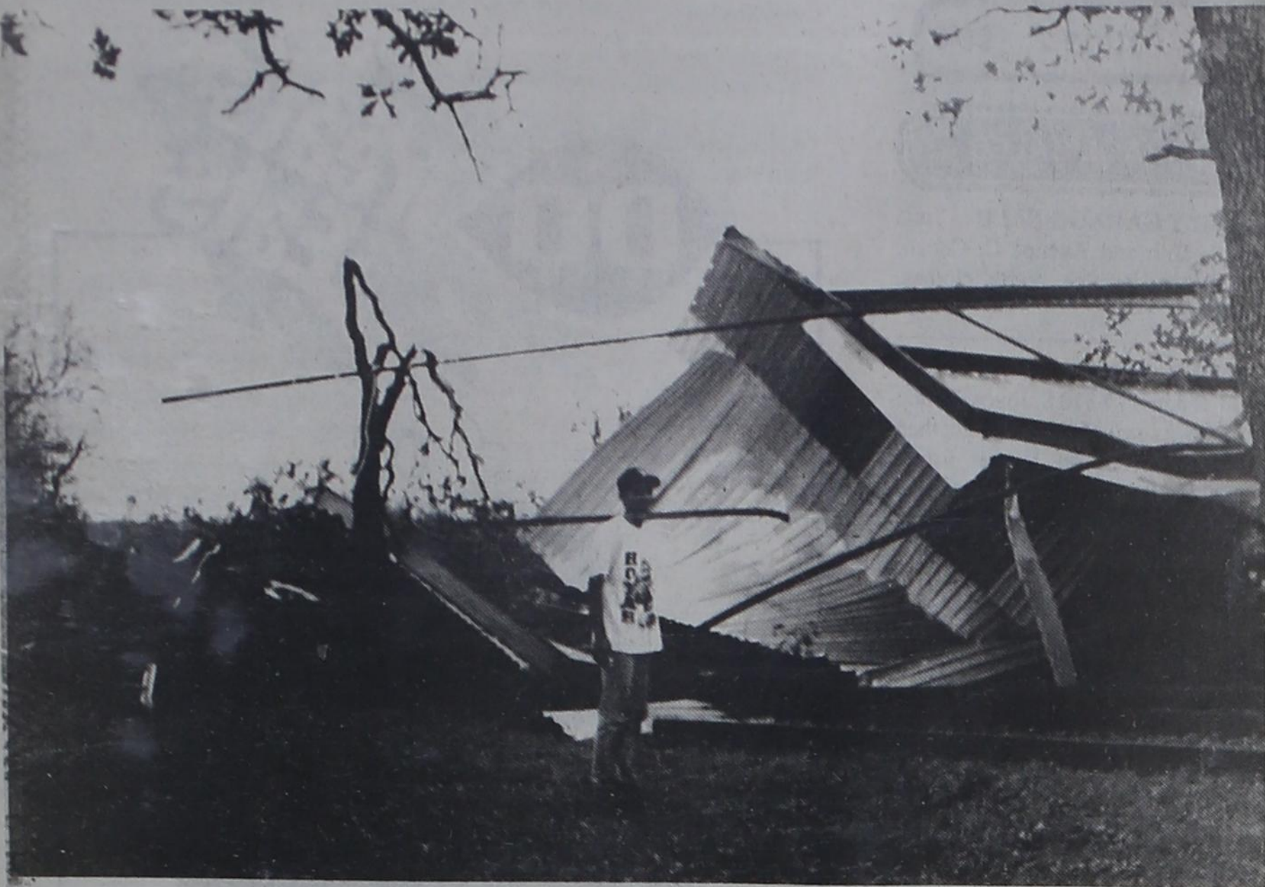
MIKE TOLLET STANDS BESIDE CRUNCHED ROOF
