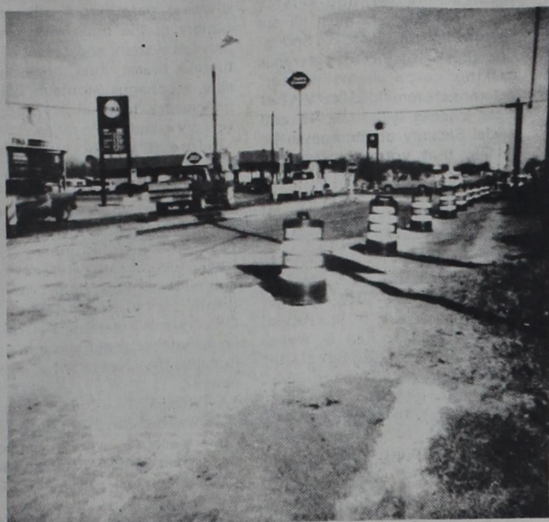
ROAD CONSTRUCTION — The intersection will be reconstructed in sections to accommodate through traffic.
