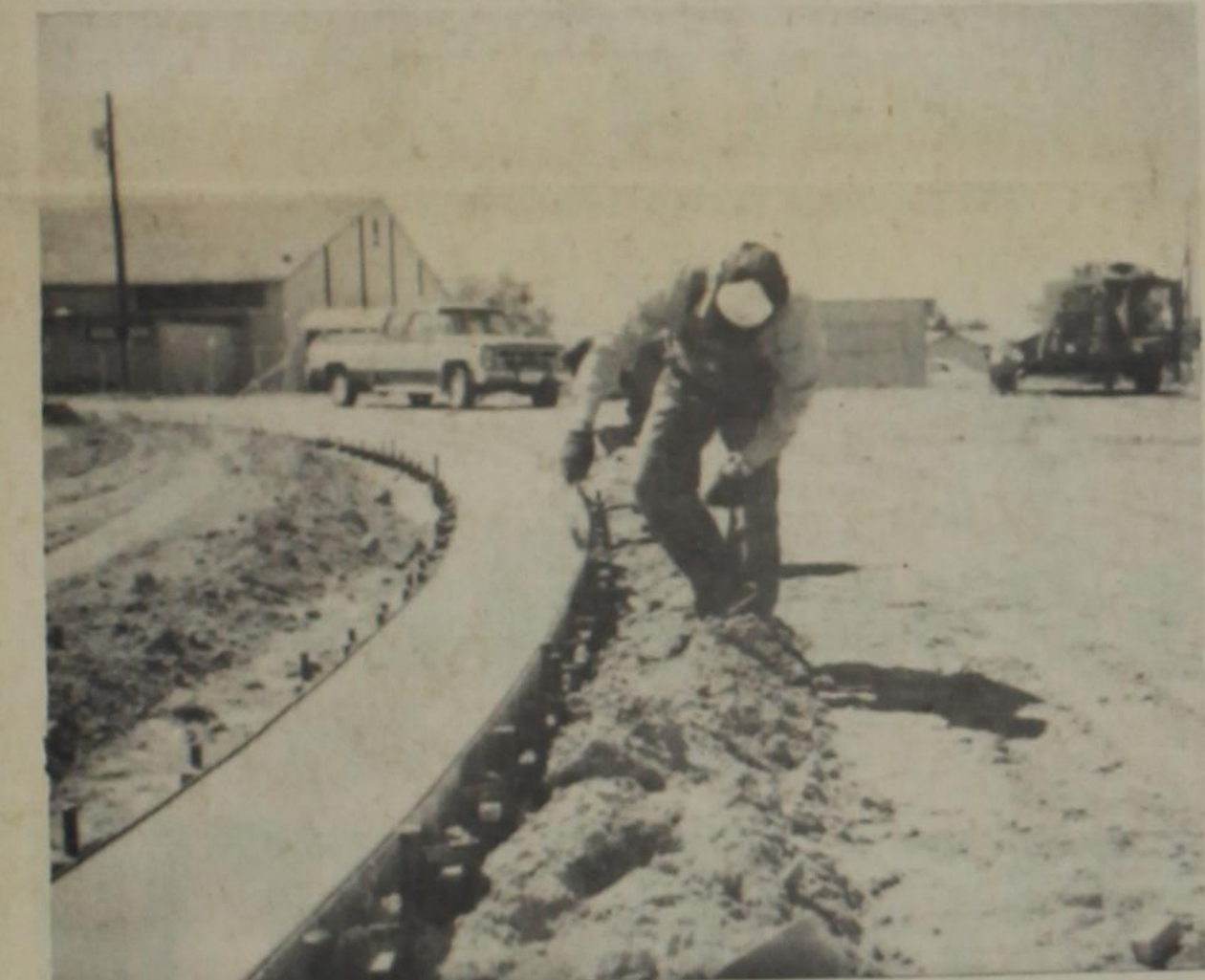
TRACK PROGRESSING — A workman pulling the edges from the form around the inside curb of the track.
