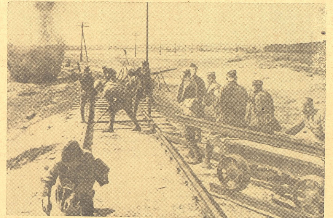
REDS UNDER FIRE—Arriving too close for comfort is Nazi shell bursting at left, but Russian engineers seem unperturbed as they re-lay bombed railroad line. However, they are not losing time.
