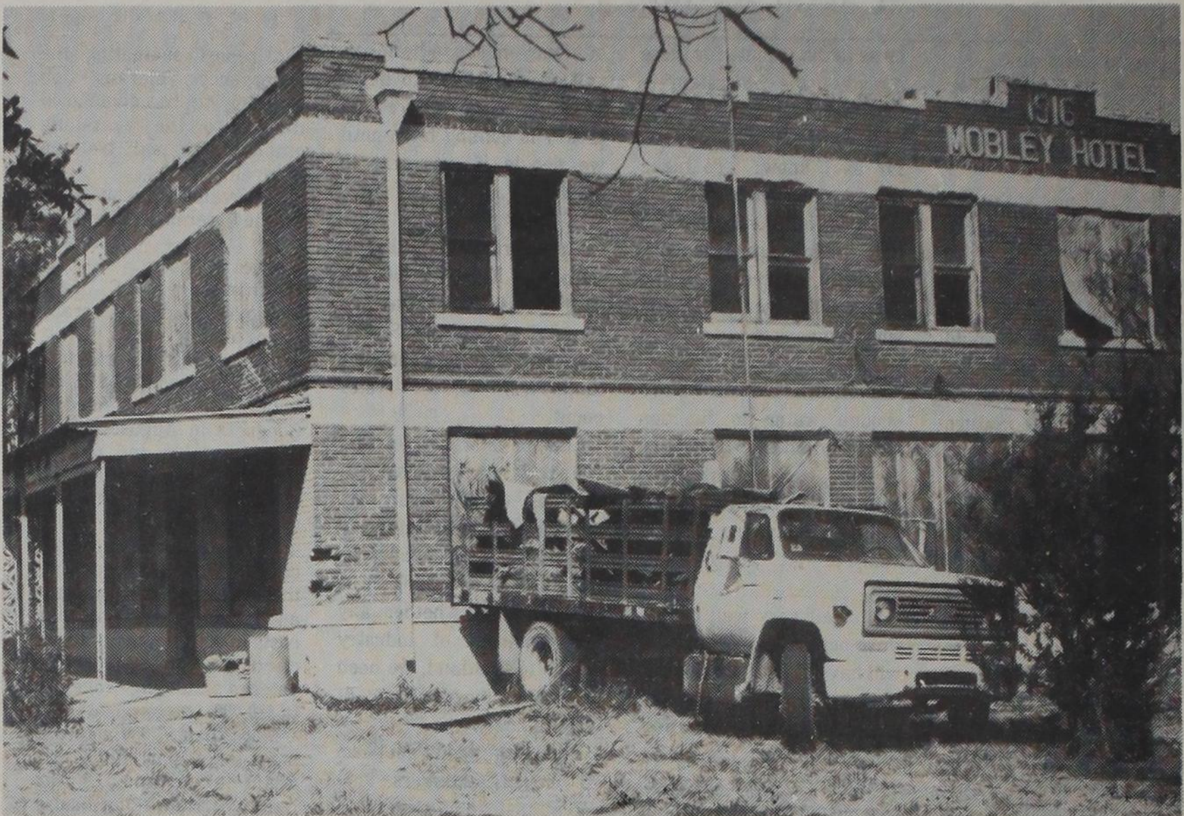
CLEANING UP- The Bennett Construction Corp. of Brownwood started work this week on the old Mobley hotel at the corner of Conrad Hilton Avenue and East 4th Street. The Mobley
