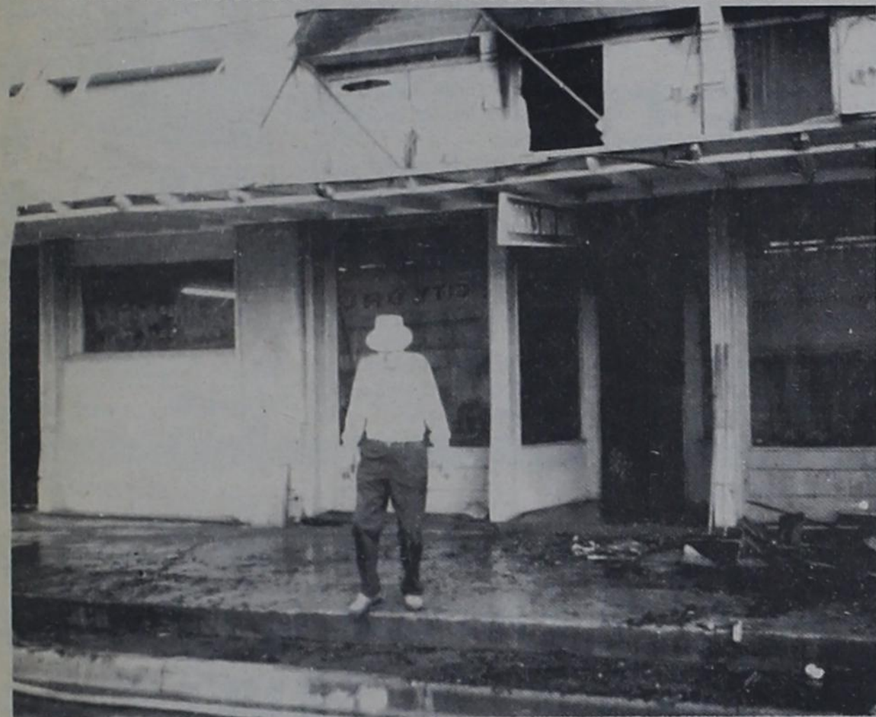
SAD OWNER —Bill Works 78, owner of Work's Dry Good store, stands outside his damaged store after fire ravaged it in an early morning fire.
