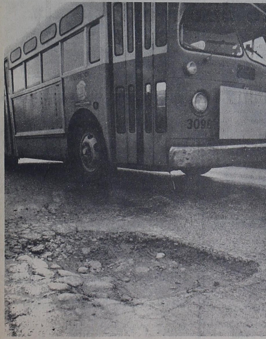
CITY BUS SWINGS WIDE Monday to avoid a deep hole in the 2700 block of 22nd Street. The hole appeared in January, when snow storms resulted in heavy street damage, but was not repaired until March 20, after Lubbock Today talked to the city public works department. (Staff photo by David Tillery)
