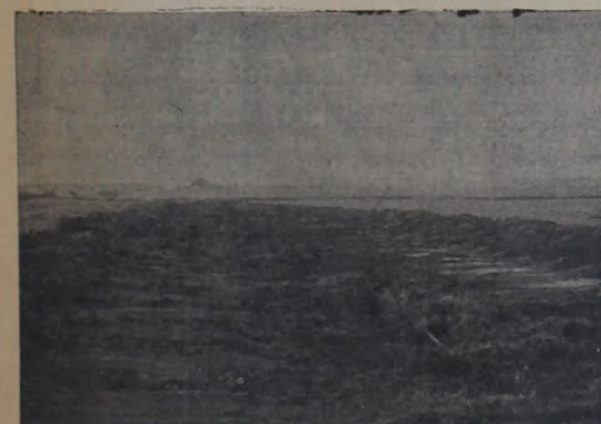
The Pierce White waterway construction is pictured as a tractor prepares the ground for seeding. This waterway, inside the Kent Creek Watershed, is part of the channel not included in the Kent Creek construction program which is to begin soon. The Soil Conservation Service and farmers are working through the Great Plains Program to accomplish this additional construction. — Photo Courtesy Briscoe County News
