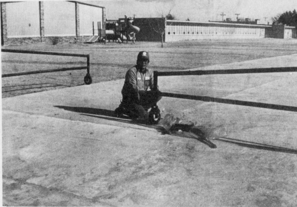
SAFETY DEVISE FOR THE DILLMAN ELEMENTARY STUDENTS---A Journal photographer happened upon Fred Bara, an employee of Muleshoe Independent School District, as he was installing one of the gates that will close off a drive through the Dillman Elementary School. The drive through (Between West 18th and 19th Streets) will be used for loading and unloading students from school buses. When not in use, the gates will be closed.
