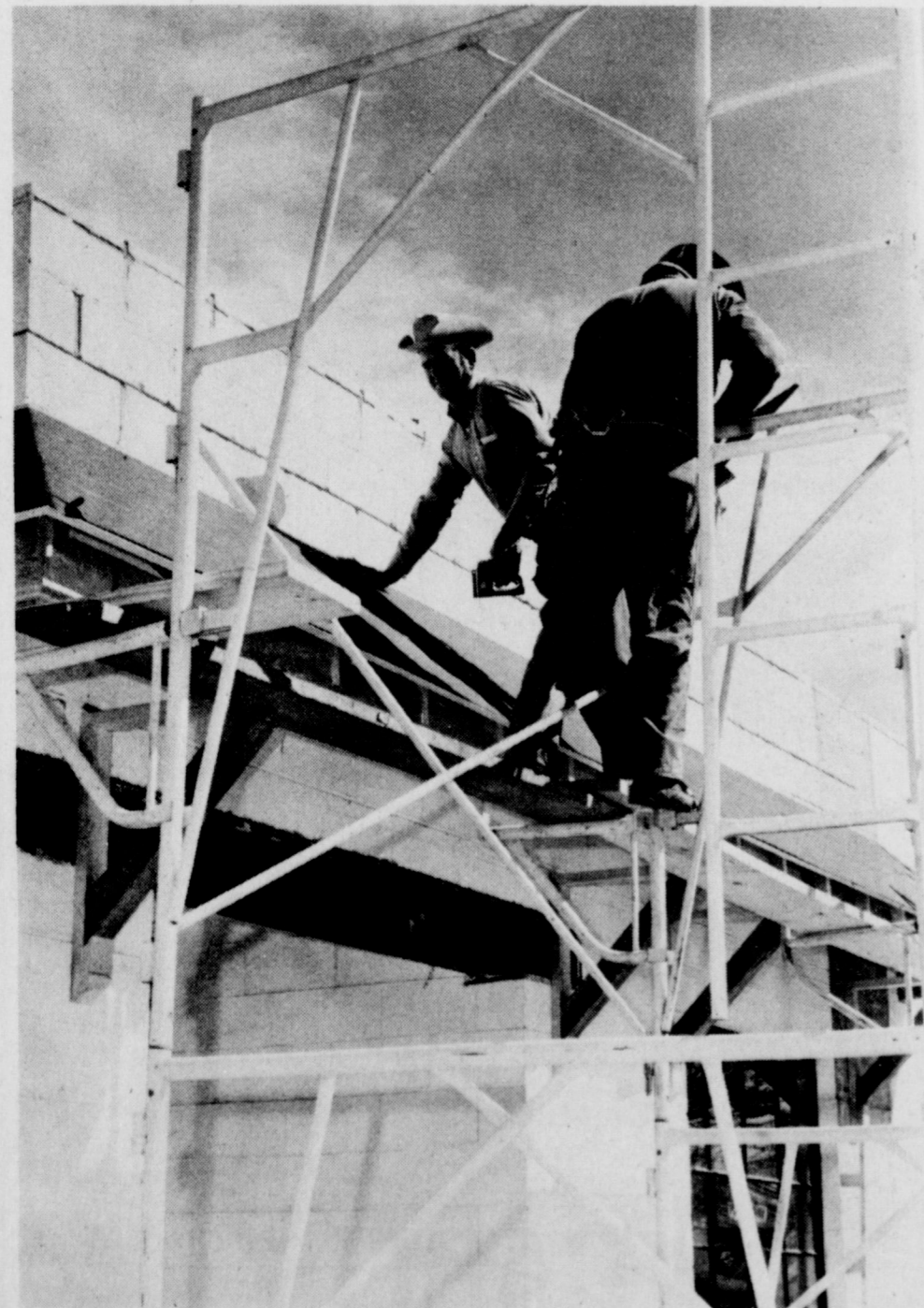
FLURRY OF ACTIVITY -- The corner of Wall and Park has been a beehive of activity recently, as workmen push to completely remodel the old post office building. It will be the home of Parker Square Savings and Loan's branch office here.
