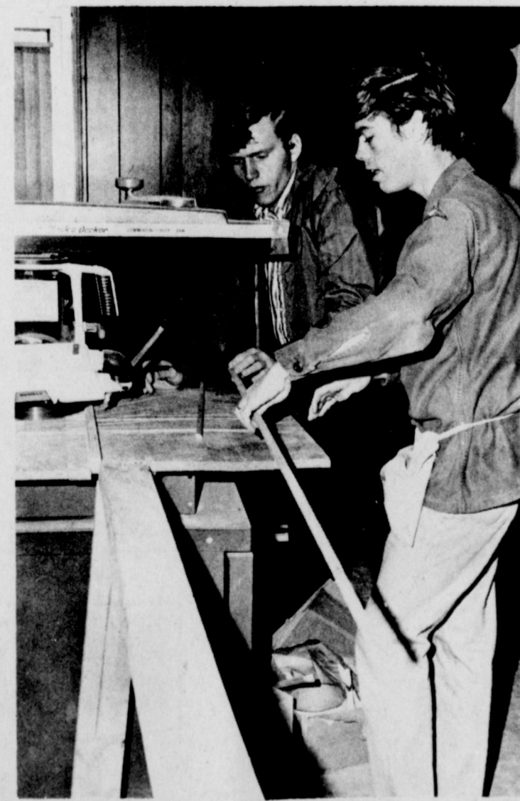
WORK PROGRESSES -- Members of the Iowa Park High building trades class last week paneled the Chamber of Commerce office, in part of the remodeling program of the Chamber. Next on the agenda, which will not be done by the students, is to paint the ceiling and carpet the floor.
