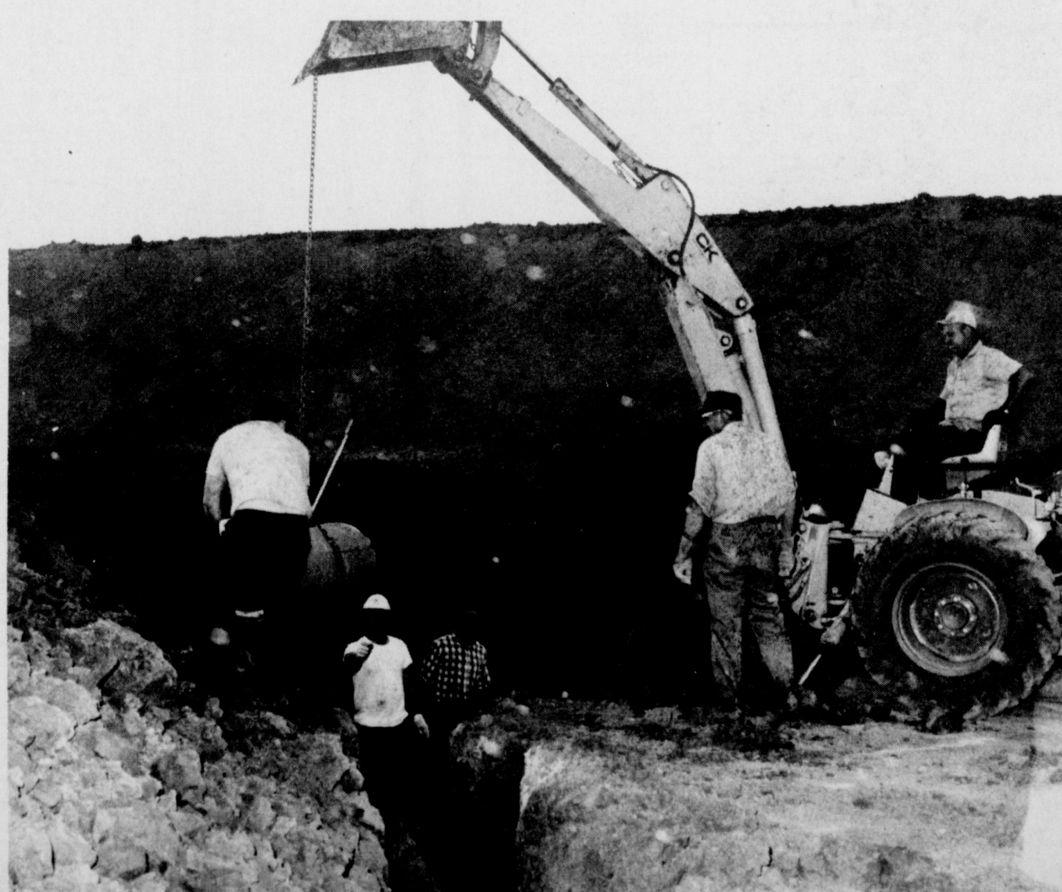
STADIUM PROGRESS--Volunteer workers are shown placing concrete drain pipe in the football stadium being constructed at the new high school. Volunteers wishing to work out their stadium seat options are asked to report Saturday morning. The schedule calls for the $129,000 facility to be completed in time for the defending state champion Hawks to open their 1970 season in the biggest "Hawk Nest" in the state.
