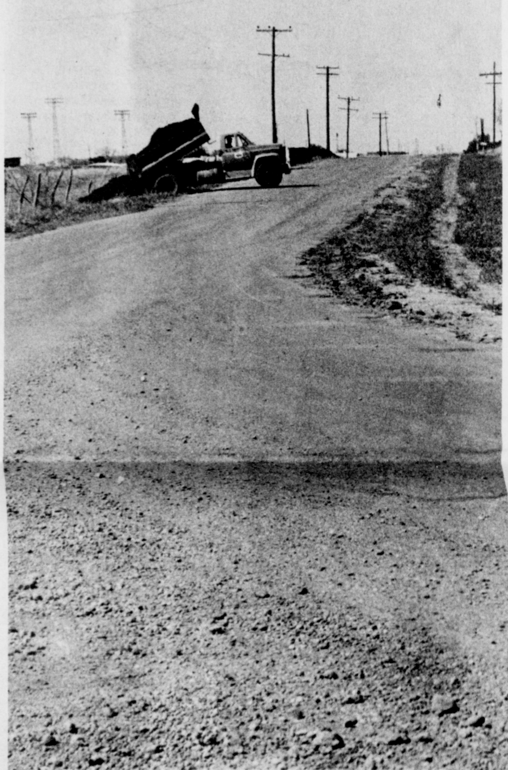
WORK IS UNDERWAY to widen Johnson Road South from its intersection with Highway West to the railroad track. Being widened by the county, trucks started filling the ditches Monday. Commissioner Buck Voyles said the project probably will extend through most of the summer, depending on demands for equipment and manpower in other areas of his precinct.
