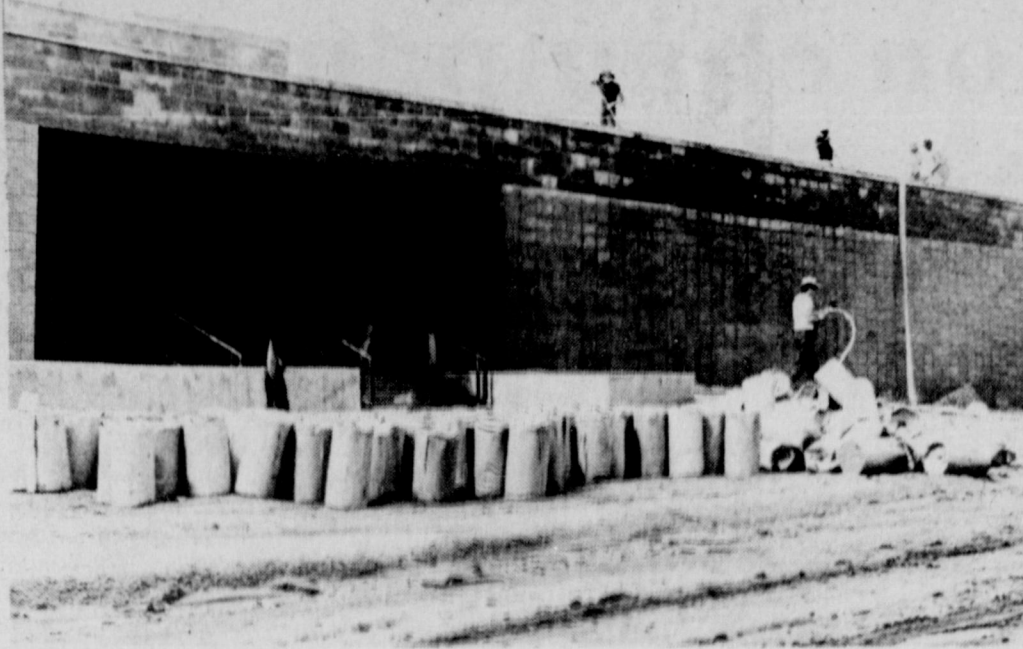
SCHOOL CONSTRUCTION - Despite recent rains construction workers at the site of Holliday's new high school have been working at a busy pace in an effort to be finished by the beginning of school next year. A view from the north shows the unfinished front of the building as crews continued work on the roof.
