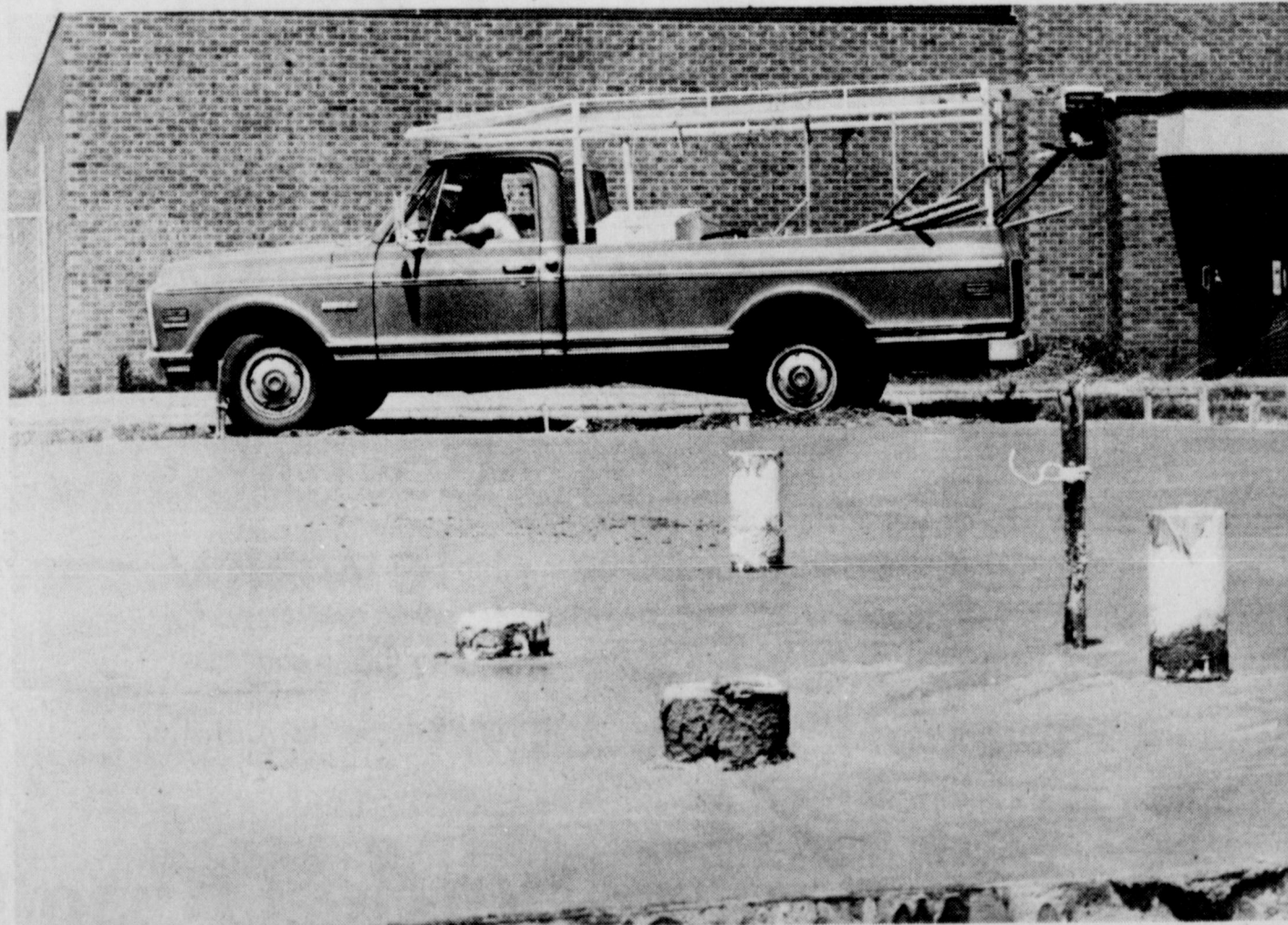
PHASE COMPLETED - Workmen load up to leave Thursday afternoon after finishing the concrete floor of the Bicentennial Swimming Pool bath house. Work was authorized to be started by the pool committee,
