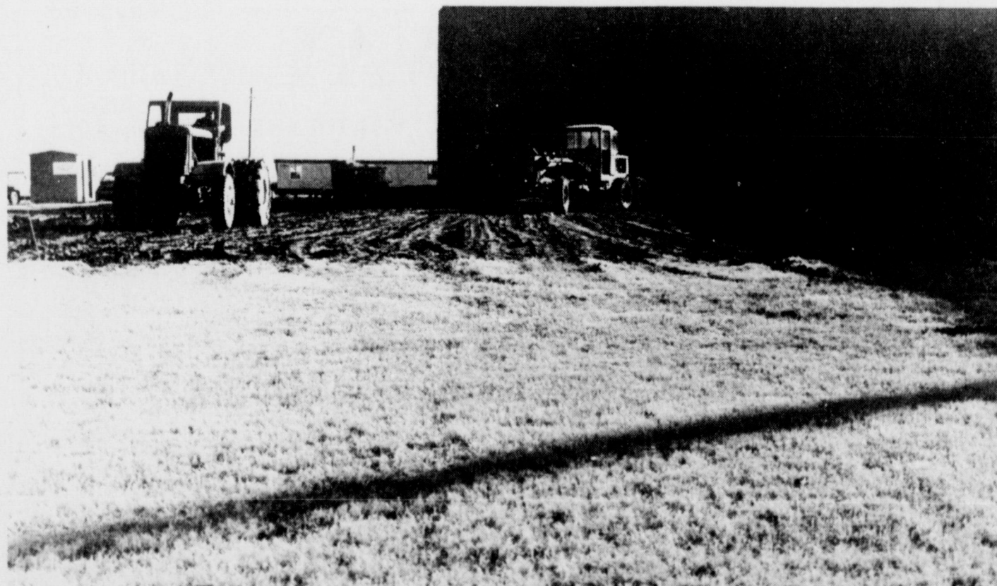
EXPANSION UNDERWAY - Crews and heavy equipment began work this week to prepare the ground around Cryovac's building, where a major expansion program is
