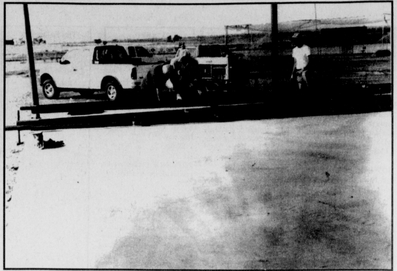
NEWEST ADDITION to the athletic facilities of Iowa Park High School is a permanent batting cage, being built by members of the Athletic Booster Club. The structure will feature a concrete floor, metal roof, and have netting on the sides.
