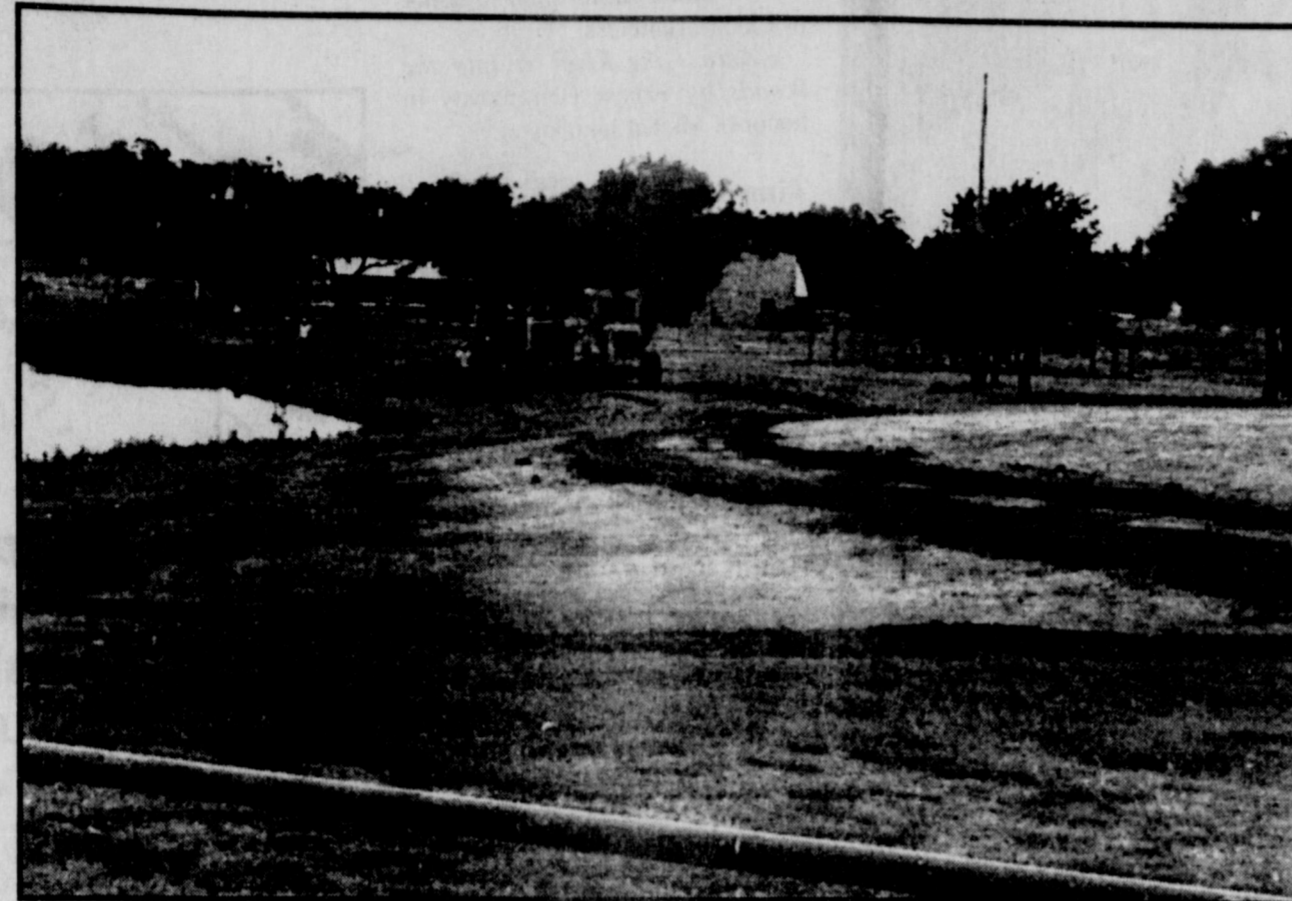
WALKING TRACK UNDERWAY - Workers began early Monday afternoon, cutting away the path of the long-awaited walking track around Gordon Lake. The facility is expected to be completed by mid-winter or early spring.
