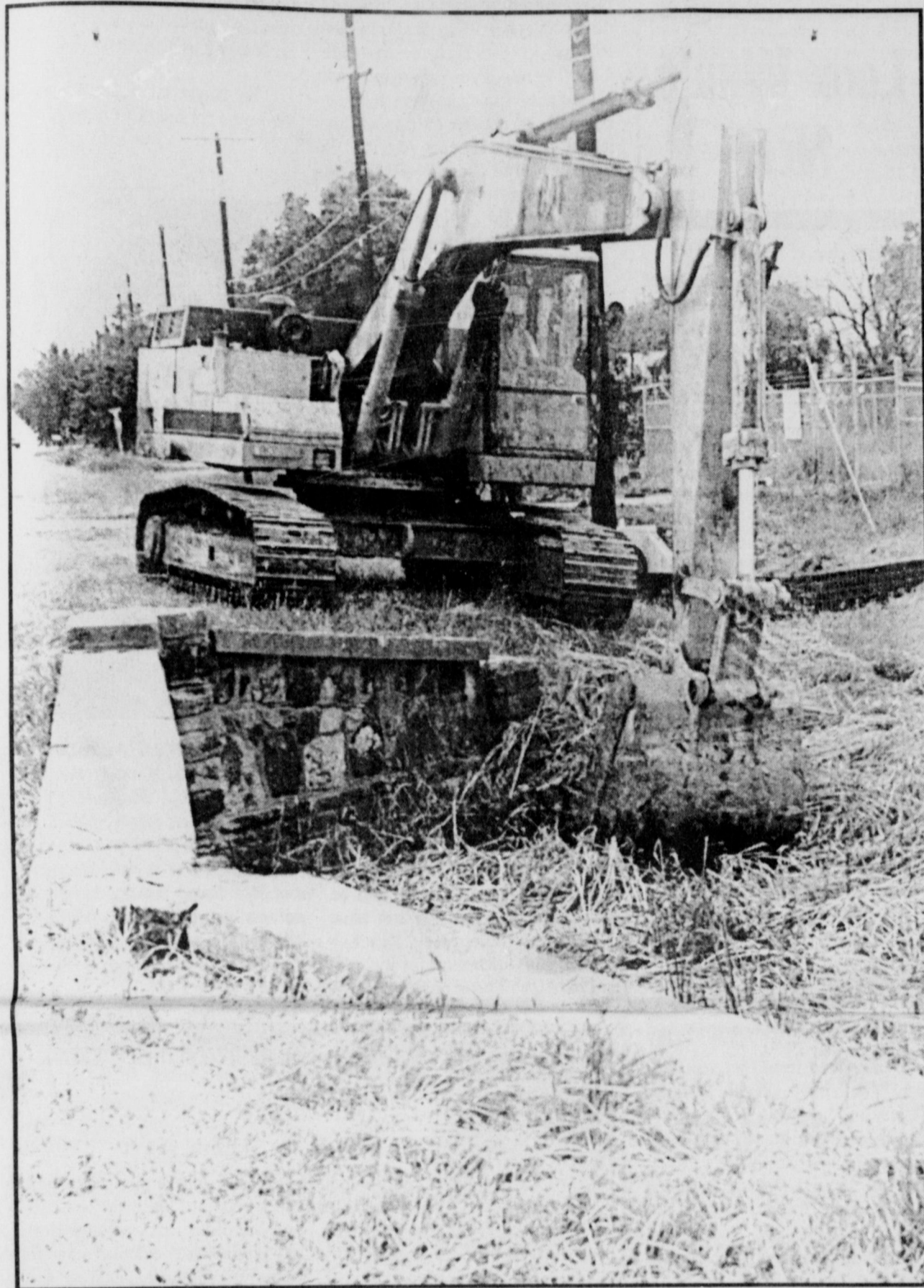
BRIDGE REPLACEMENT - Work was begun Monday to replace the half-century-old bridge over the creek at Victoria and Texas. The project is the initial phase of completely rebuilding Victoria, from Cash to the Access Road.
