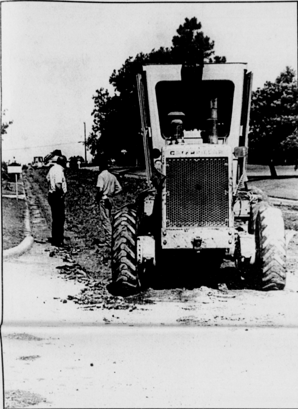
STREET WORK PROGRESSING - The city's street crew was busy tearing out the old asphalt surface in the 600 and 700 blocks of Cornelia this week, in preparation of relacing it. Meanwhile, asphalt is to be laid either Friday or next Monday in the 200 and 300 blocks of West Park, according to Belvin Lytle, public works director.
