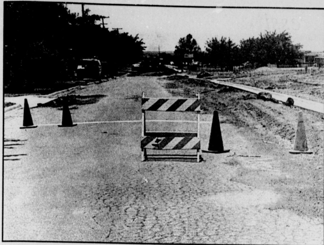
LONG-AWAITED PROJECT UNDERWAY - City workers have begun the task of taking out the old, original asphalt paving on North Third Street, with the intention of widening and resurfacing it, as well as installing curb and gutter. When the city rebuilt the street from West Highway to Rebecca some eight years ago, the project was terminated for lack of funds. Administrator Mike Price says he hopes to have the project completed, or near completion, by the time classes begin at Kidwell Elementary.
