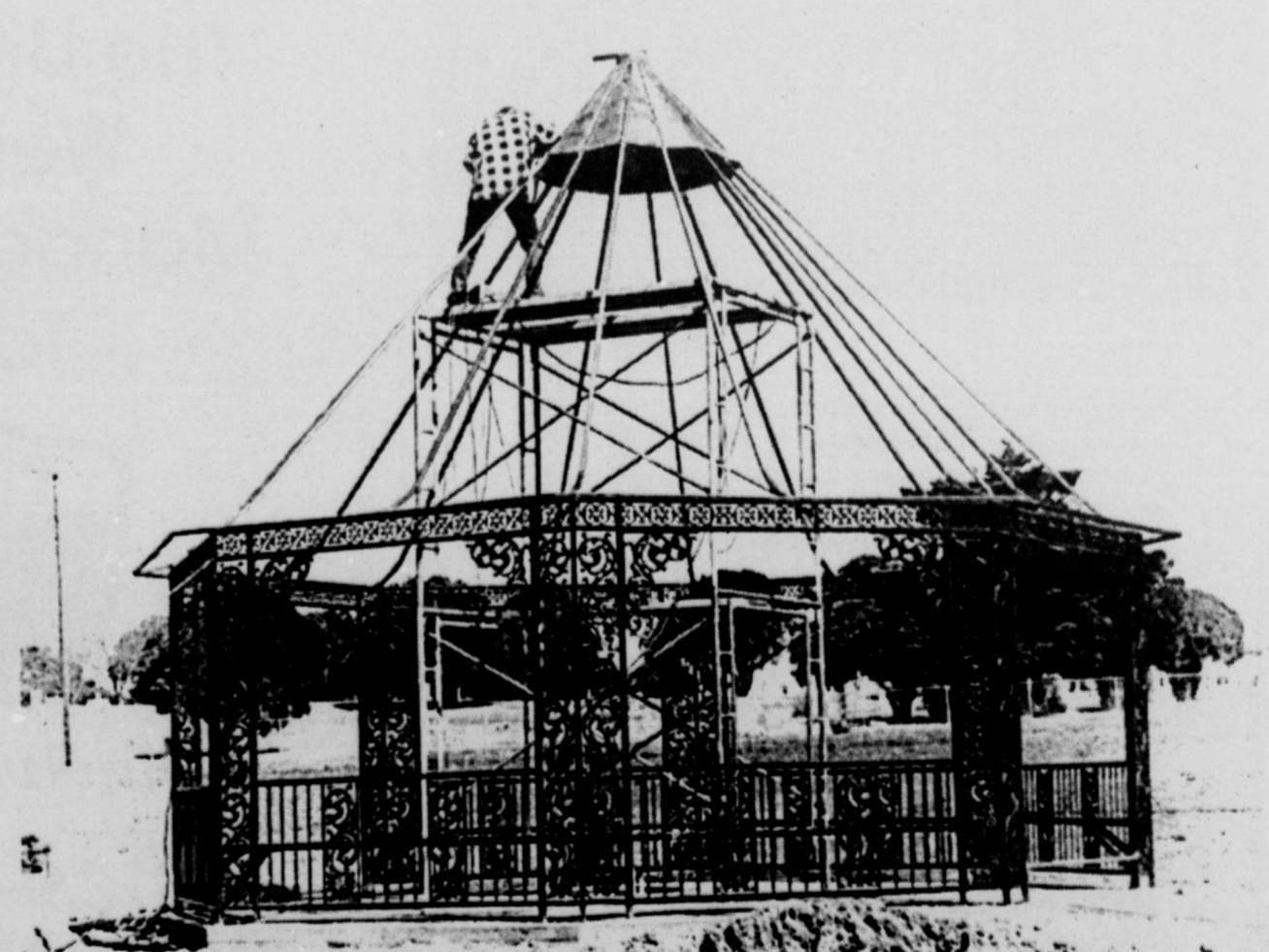
BEAUTIFICATION UNDERWAY - A wrought iron gazebo is being constructed on land between US 287 and Highland Cemetery, and once it and grass seeding is completed, the area will be considerably more attractive than when it was covered with mesquite trees. The land was donated to the cemetery by the W.F. George Estate, and Highland Cemetery Association has undertaken the improvement project.
