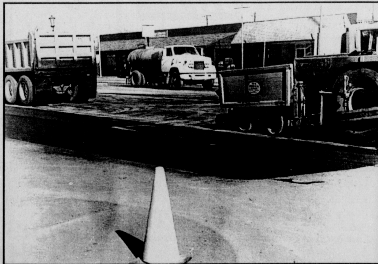
PROJECT COMPLETED - After a lengthy waiting period, crews worked Tuesday and Wednesday to overlay existing pavement and lay on new pavement in the 300 block of North Wall. The work completed overlaying of all downtown business streets, and for the first time, defined the street and parking areas in that particular block, complete with newly-installed gas lights.
