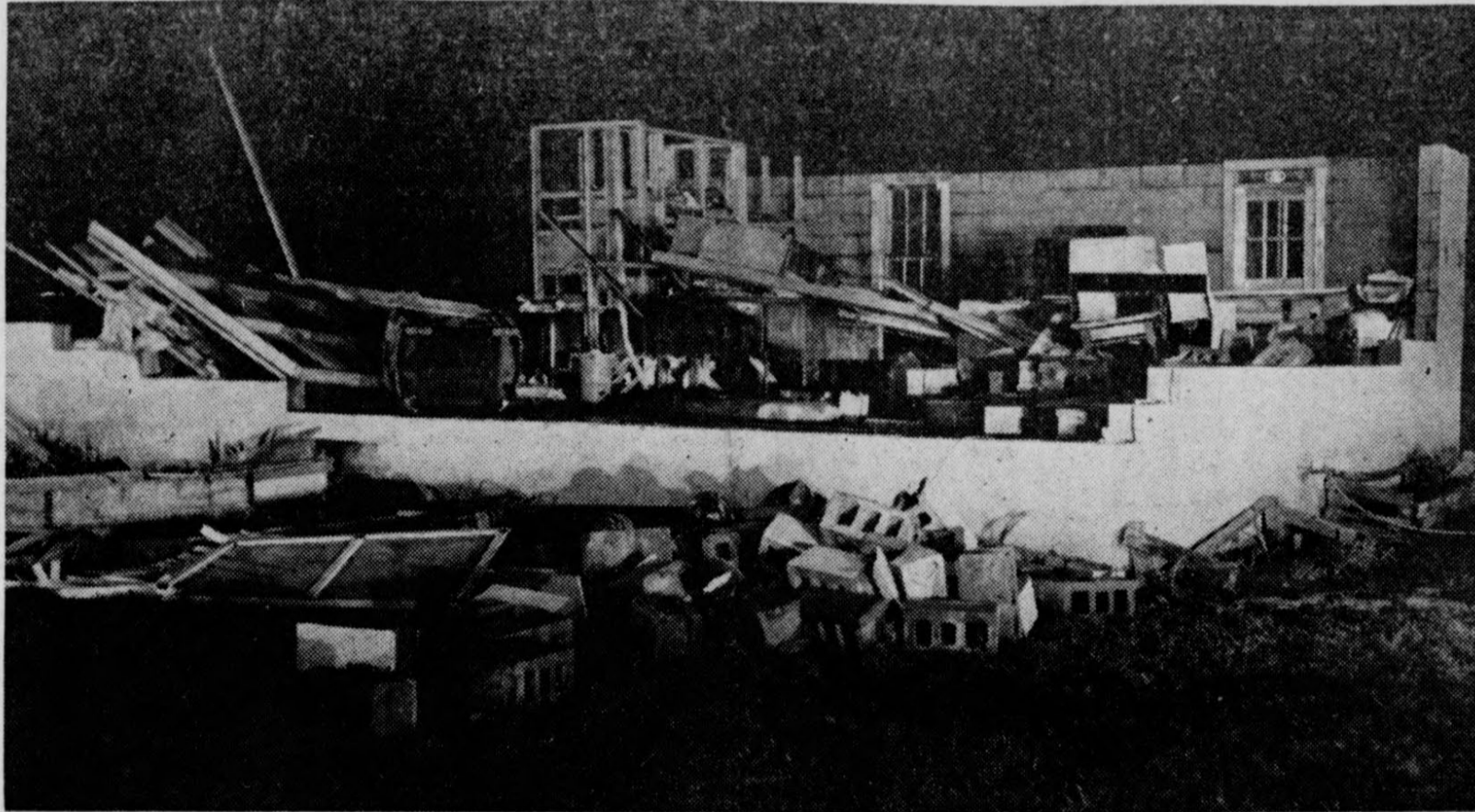
Wichita Record News photographers took this shot of the J. D. Harrell home shortly after the storm Tuesday night
