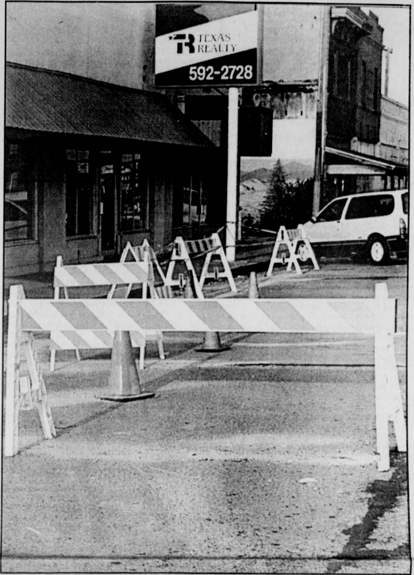
GETTING THINGS READY - City street workers for the past few weeks have been patching cracks in downtown concrete pavement, in preparation for an asphalt overlay. The overlay project is tentatively scheduled this weekend, according to Belvin Lytle, public works director. The schedule includes: surfacing Yosemite from West Highway to Bank, and the 200 and 300 blocks of west-bound West Park on Saturday; Wall from East Highway to Bank, 100 West Cash and east and west lanes of 100 West Park, on Sunday. Lytle emphasized that weather conditions must be favorable, or the work will be postponed until the following weekend.
