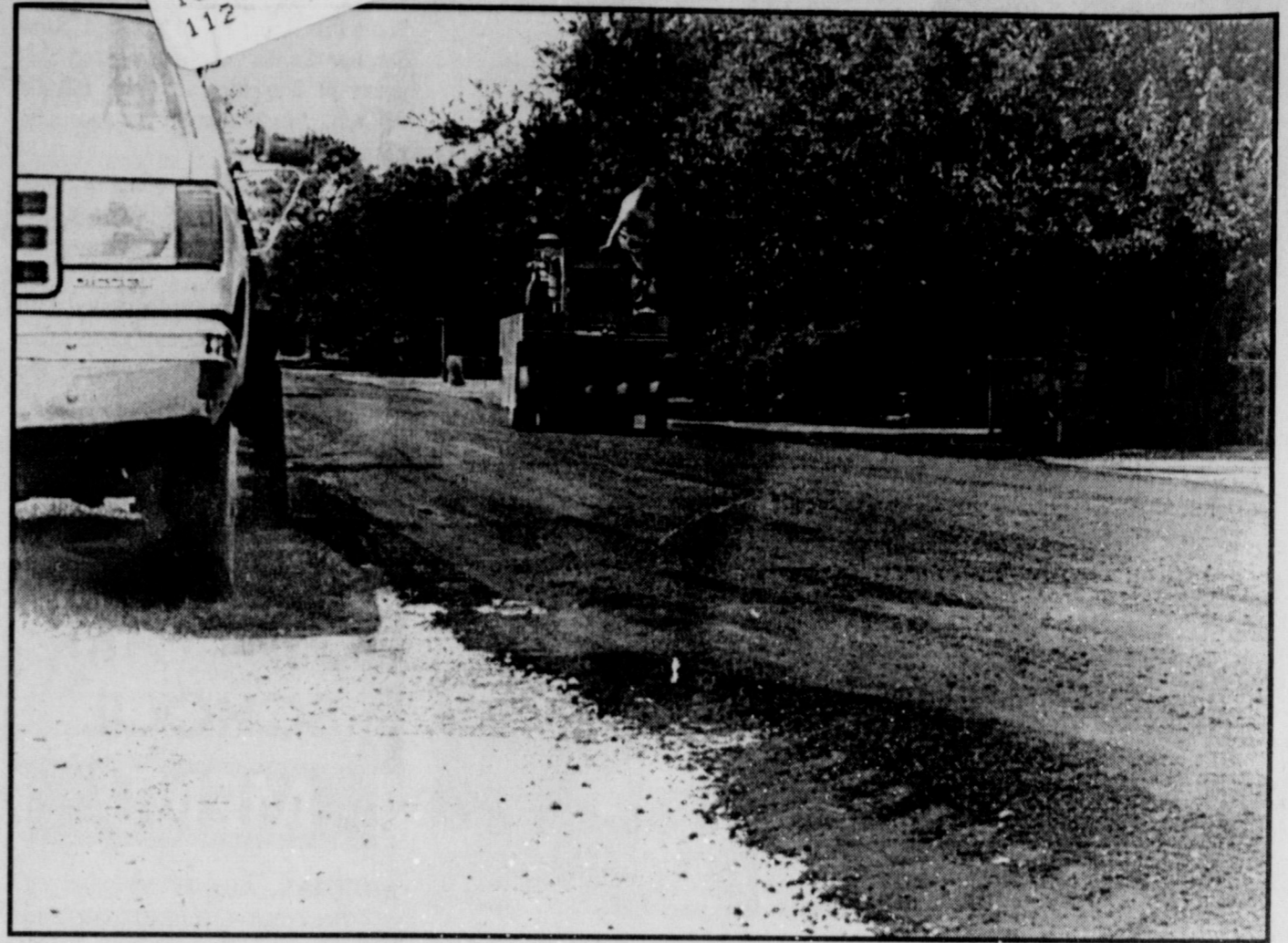
STREET WORK PROGRESSING - Crews applied an asphalt overlay this week on Pasadena, as part of the city's summer street improvement project.
