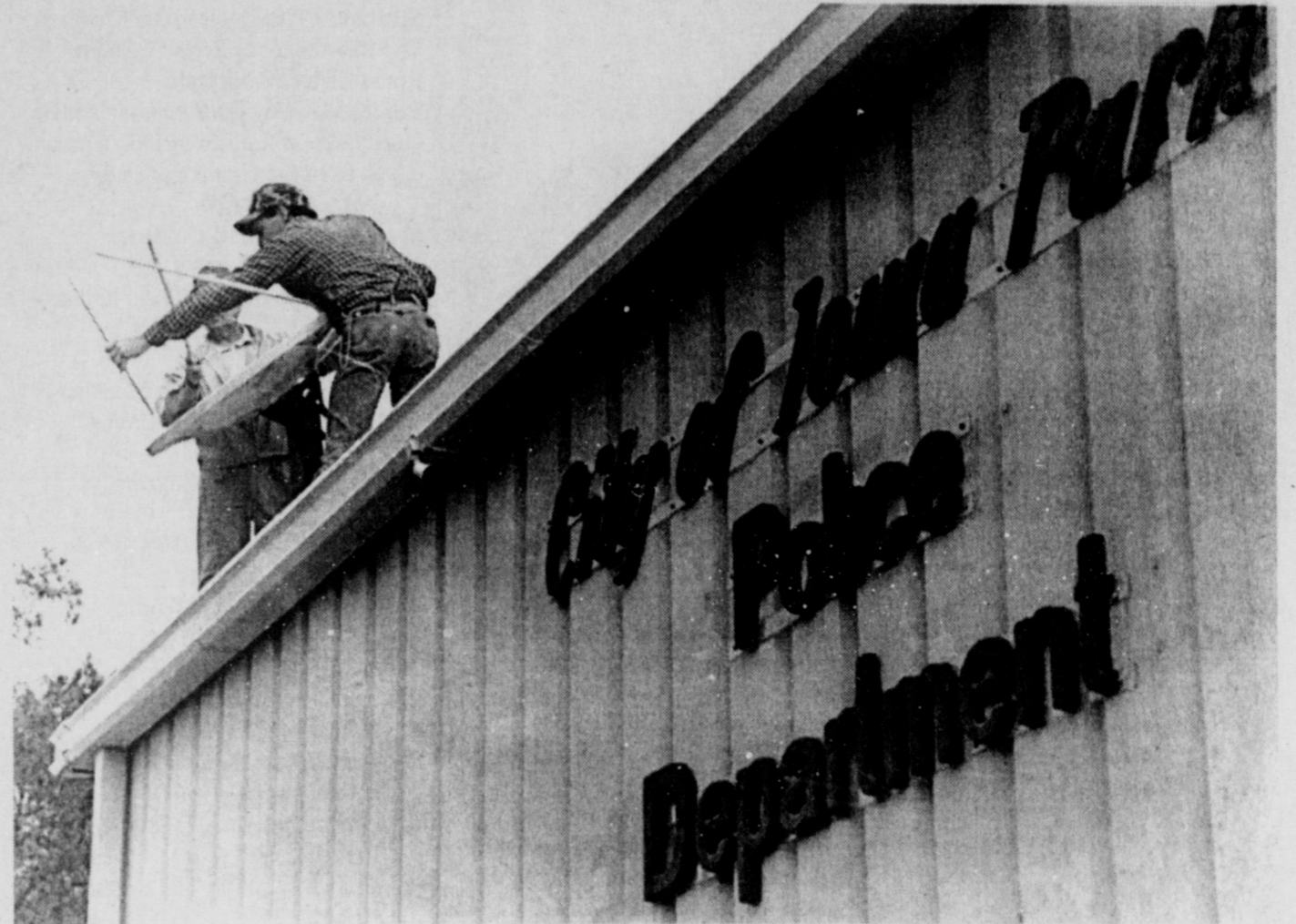
HELP IS HERE for weather spotters during storms. A satellite receiver, monitor and control equipment were installed this week at the Iowa Park police station. The equipment provides local forecasting, radar coverage and also satellite pictures of cloud formations.
