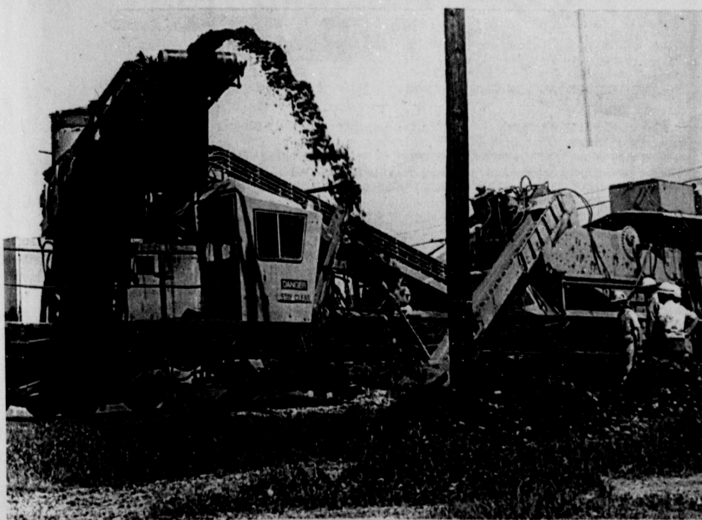
MONSTROUS MACHINE - Burlington Northern Railroad crews were busy doing major renovation of the lines through Iowa Park this week. They began earlier this month at Wichita Falls and are progressing westward. This machine is capable of lifting the track, taking out all the rock base and replacing it with new rock, as it moves slowly through the day.
