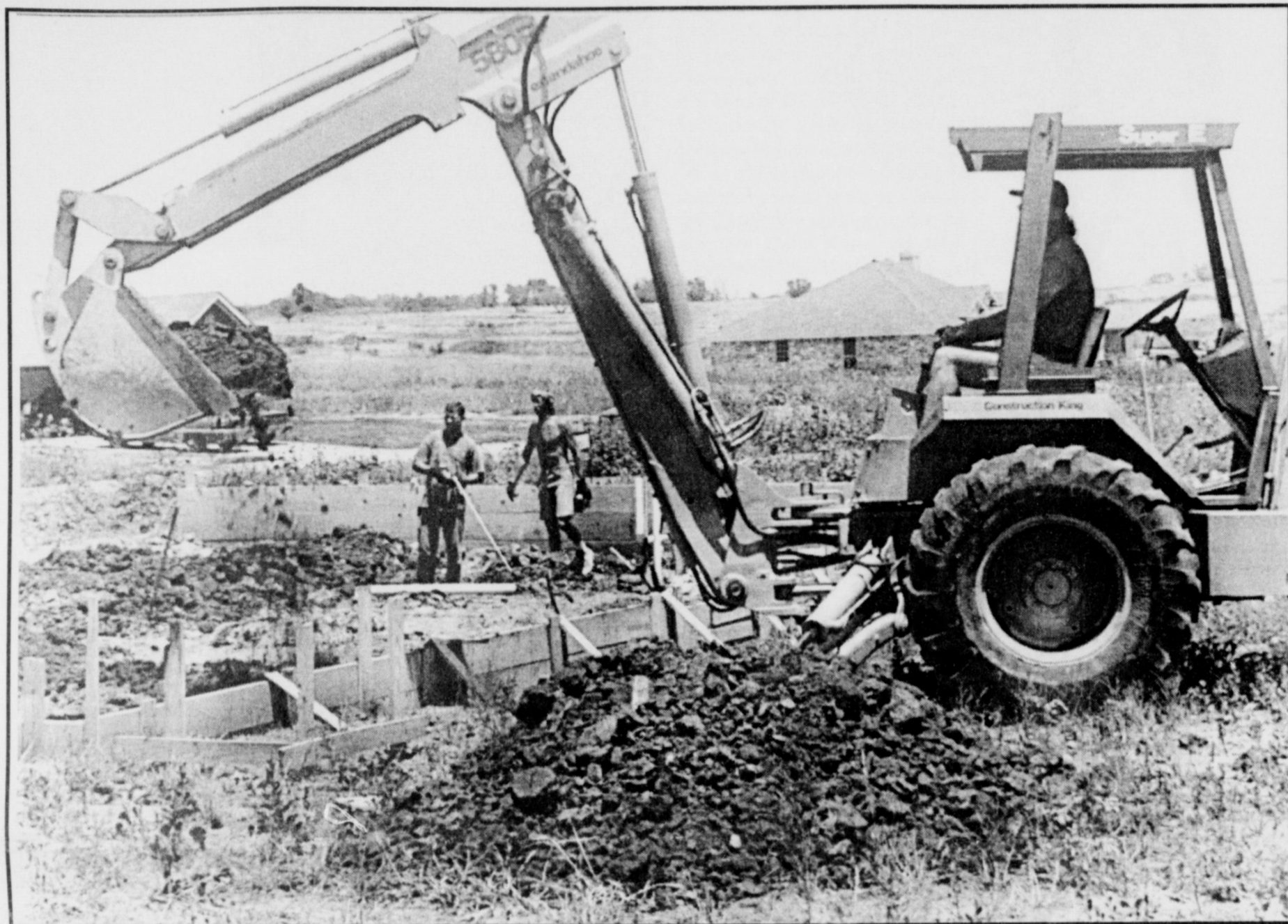
WORKERS DIG FOUNDATION ON ONE OF THREE NEW HOMES IN PARK PLACE ADDITION
